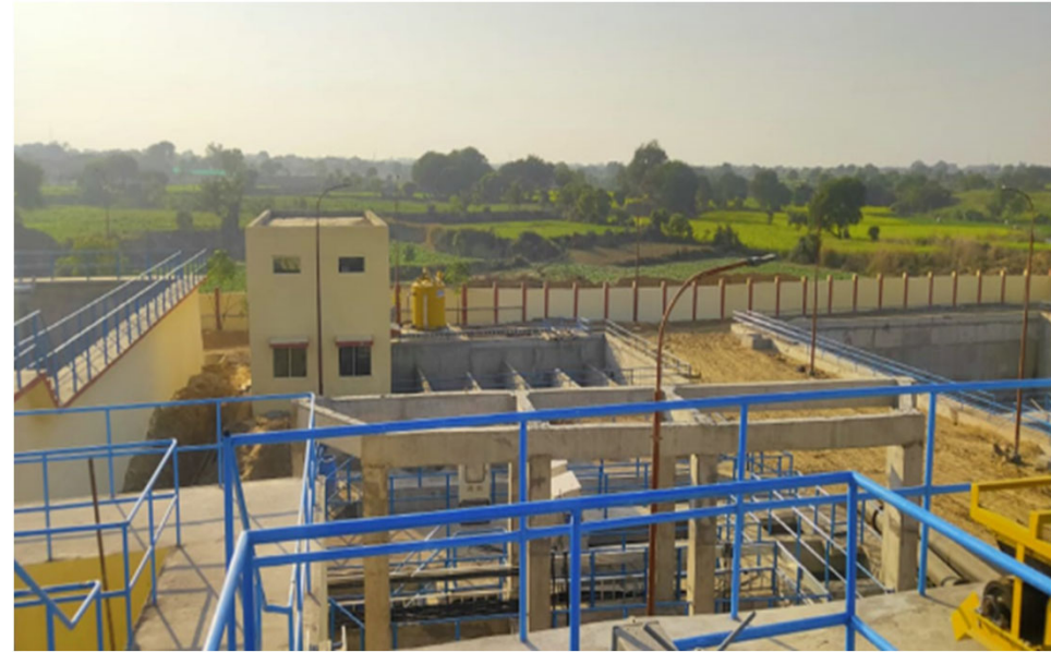
12 MLD STP IN BHIND
