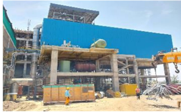
Air Cooled Condenser
